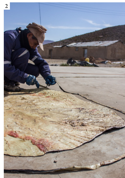
1: Crowning of a perimeter wall 2: Cutting of the cowhide to make the laces used in the roofing
