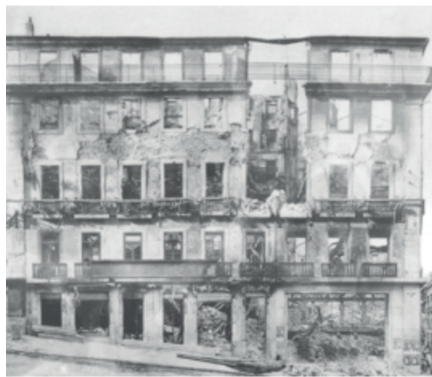
Fig. 1.3. Chiado after the fire.
