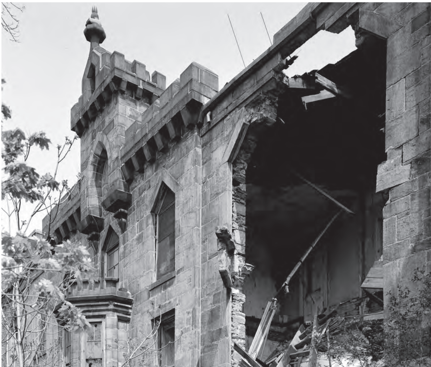
Western façade showing a partial collapse of the wall, Library of Congress, 1983. ( https://theruin.org/history ).
