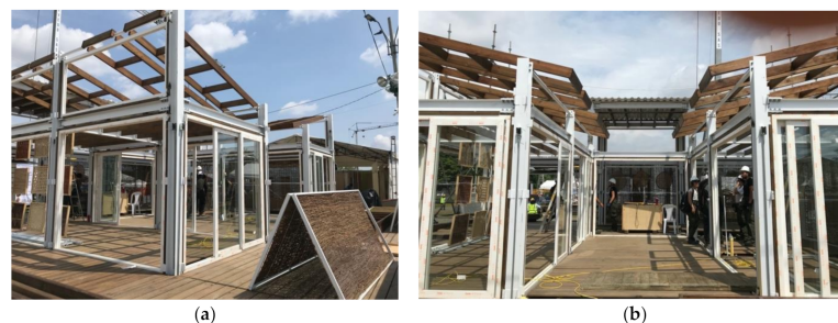
Figure 5. The PEI Maquina Verde’s House construction: (a) on the left the floor and the roof wood beam installation; on the right corner the shading device before the installation, it has made up with vegetal texture installed above a metal frame; (b) the PVC windows installation over the steel structure, the window-to-wall ratio is 80%.
