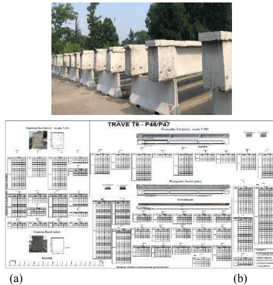
Fig. 2. (a) Beams on the inspection site. (b) Example of damage inspection sheet.
