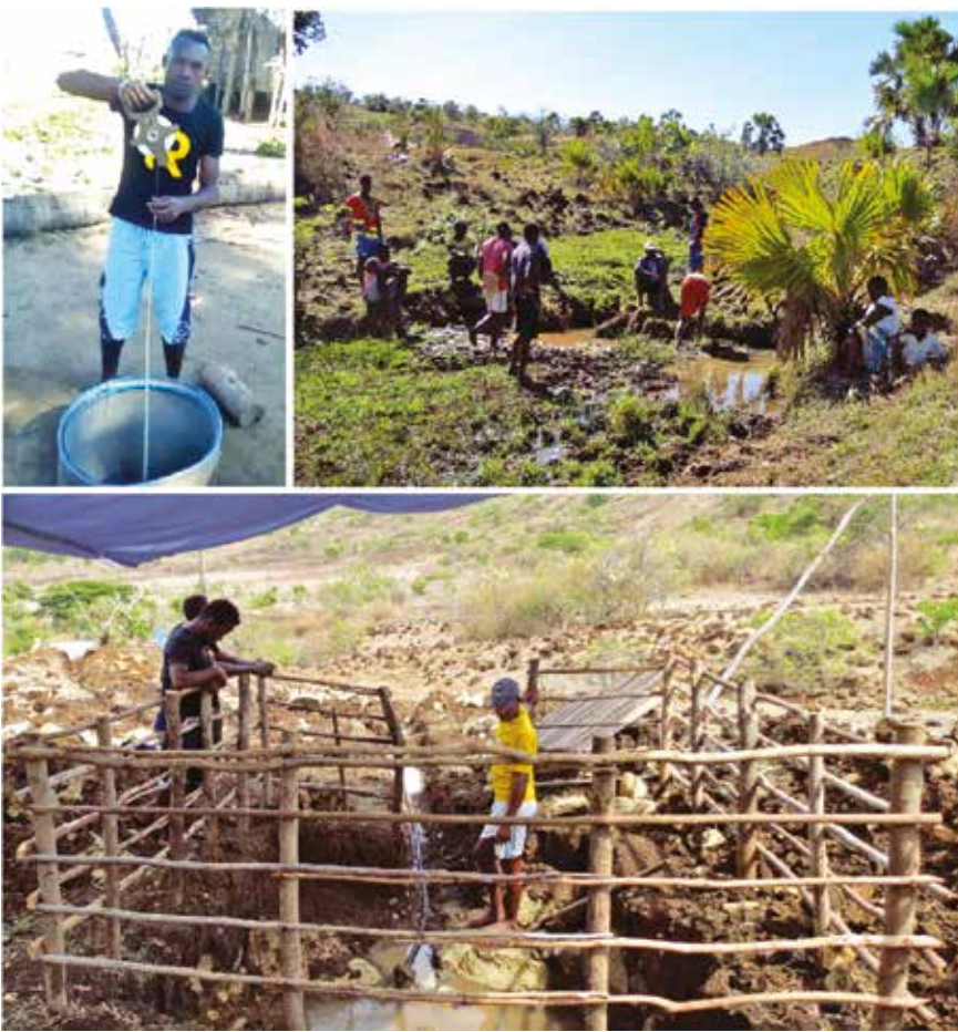
Fig. 4 – Photos taken on Nosy Mitsio island. From top left: a local man measures the well depth; the source WS01 at its natural state; locals engaged in the construction of the water catchment at source WS01.
