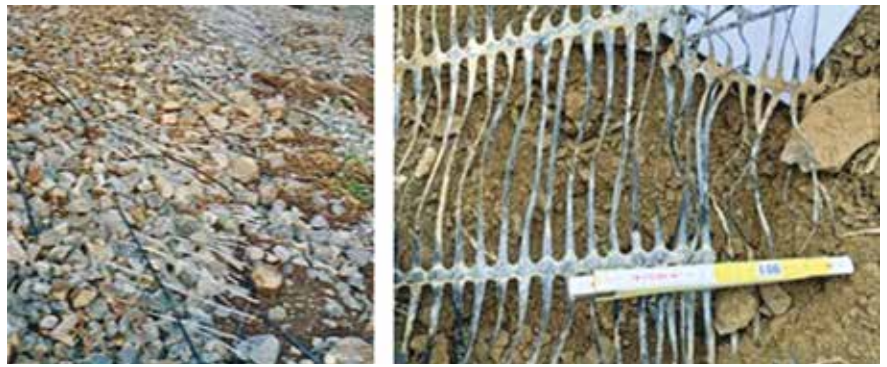
Fig. 2 – Typical tension cracks formed inside the disassembled body of the embankment: on the left woven geogrids elongated in collapsed earth support structure; on the right extruded geogrid elongated after the impact of the block in a protection embankment. Same graphical scale. (credits personal archive C.Oggeri).
