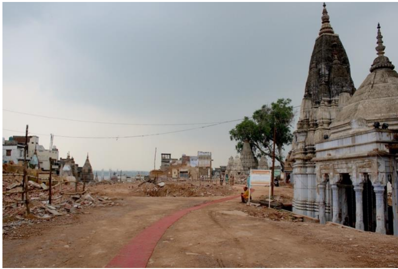
Figure 37 Another area cleared by the demolitions, with the temples on the right and the debris of demolished houses on the left, November 2019. Author's picture.
