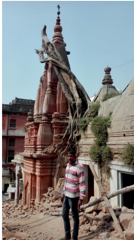
Figure 12 My acquaintance showing me the area demolished by the KVSAD Project. Author's picture.
