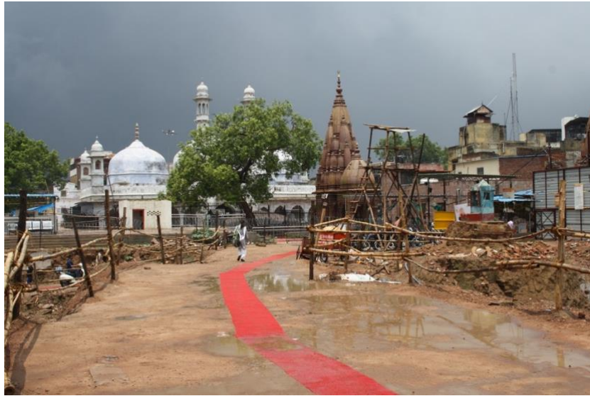
Figure 41 The demolished area stretching towards the Gyan Vapi Mosque compound, which is now more visible, November 2019. Author's picture.
