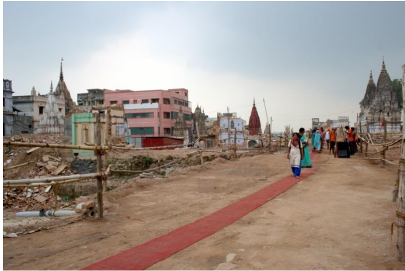
Figure 35 The corridor area created by the KVSAD Project by demolishing the existing fabric, November 2019. Author's picture.
