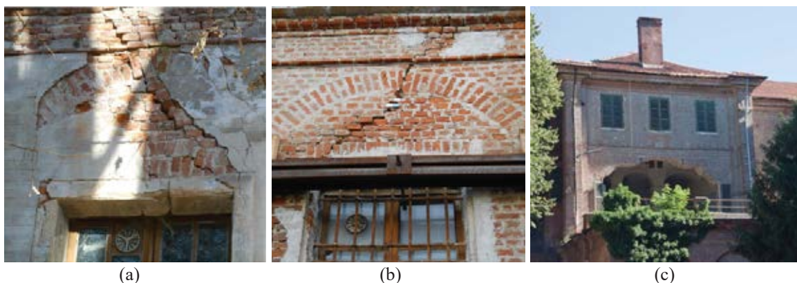
Figure 1: (a-b) some cracks on the various facade of the building (2015); (c) collapse of a portion of the southern façade (2016).
