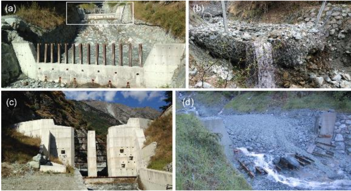
Fig. 2 The structural mitigation works along the Grand Valey torrent: (a) the two filter barriers at the Pèrriere hamlet; (b) the steel net barriers; (c) the slit-filter barrier at Tromen; (d) the barrier at Pèrriere (white rectangle in Fig. 2a) that collapsed in 2014. The position of each of these structures is indicated in Fig. 1 (photos courtesy of the Aosta Valley Autonomous Region).
