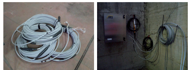
Fig. 5 - Water temperature measuring chain (PT1004/Pt) installed in S2-control piezometer of the Politecnico of Torino open-loop GWHPs
