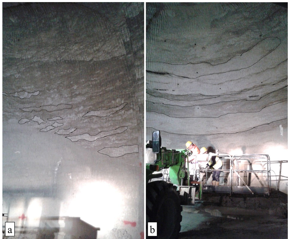
Fig. 27 Excavation faces in underground tunnels in branching selenite gypsum with different macro-textural features. a Small gypsum nodules in a predominant fine matrix. b Big coarse gypsum branches with lower concentration of finer matrix
