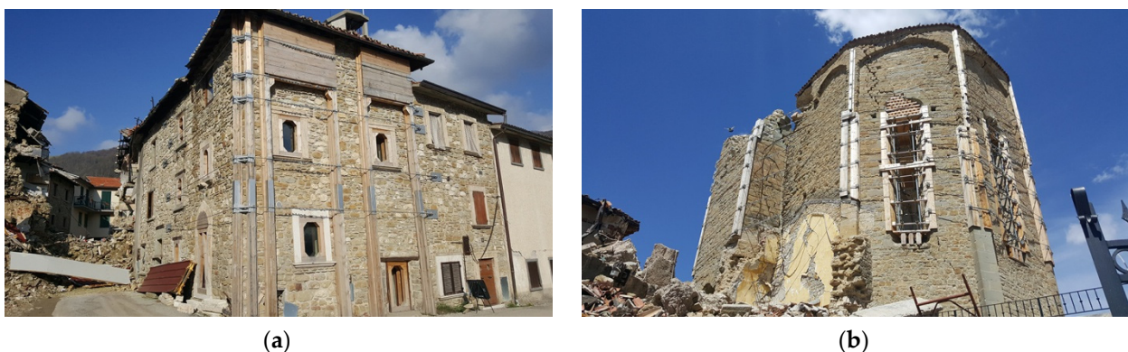
Figure 2. (a) Damaged masonry buildings in the area around the epicenter of the 2016 Central Italy earthquake; (b) St. Francesco church in Amatrice, damaged by the same earthquake.
