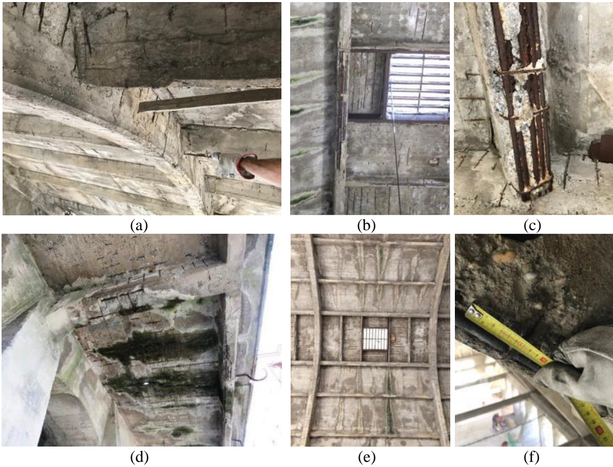
Figure 7: Damage and degradation on the building: (a) exposed rebars on the AR; (b-c) exposed rebars and detachments of concrete of the joists and roofing panels; (d) water staining and bio growth on the elements of the outdoors shelter; (e) a general view of the interior of the Paraboloid showing water staining and bio growth on the roofing panels; (f) a detail of the exposed rebars of a parabolic arch.
