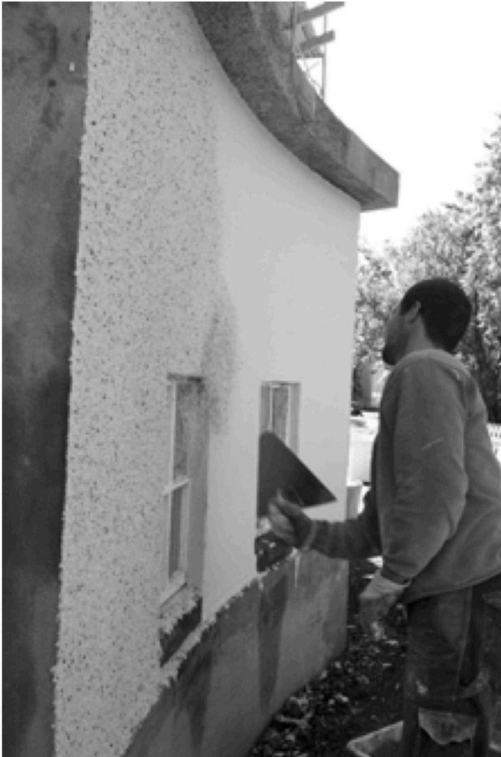
Fig. 39 – The application of steining with a trowel. Ári Trausti Guðmundsson, and Flosi Ólafsson, Steinuð Hús , 32.
