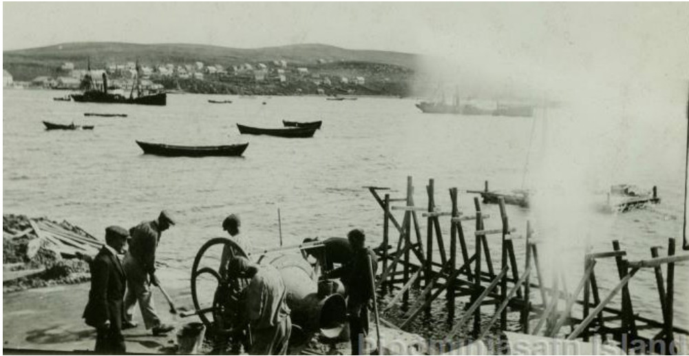
Fig. 35a – Concrete mixer in use during the works for a pier in the harbour of Hafnarfjörður. Photo by engineer Thorvald Krabbe, 1912. Þjóðminjasafn Íslands/National Museum of Iceland
