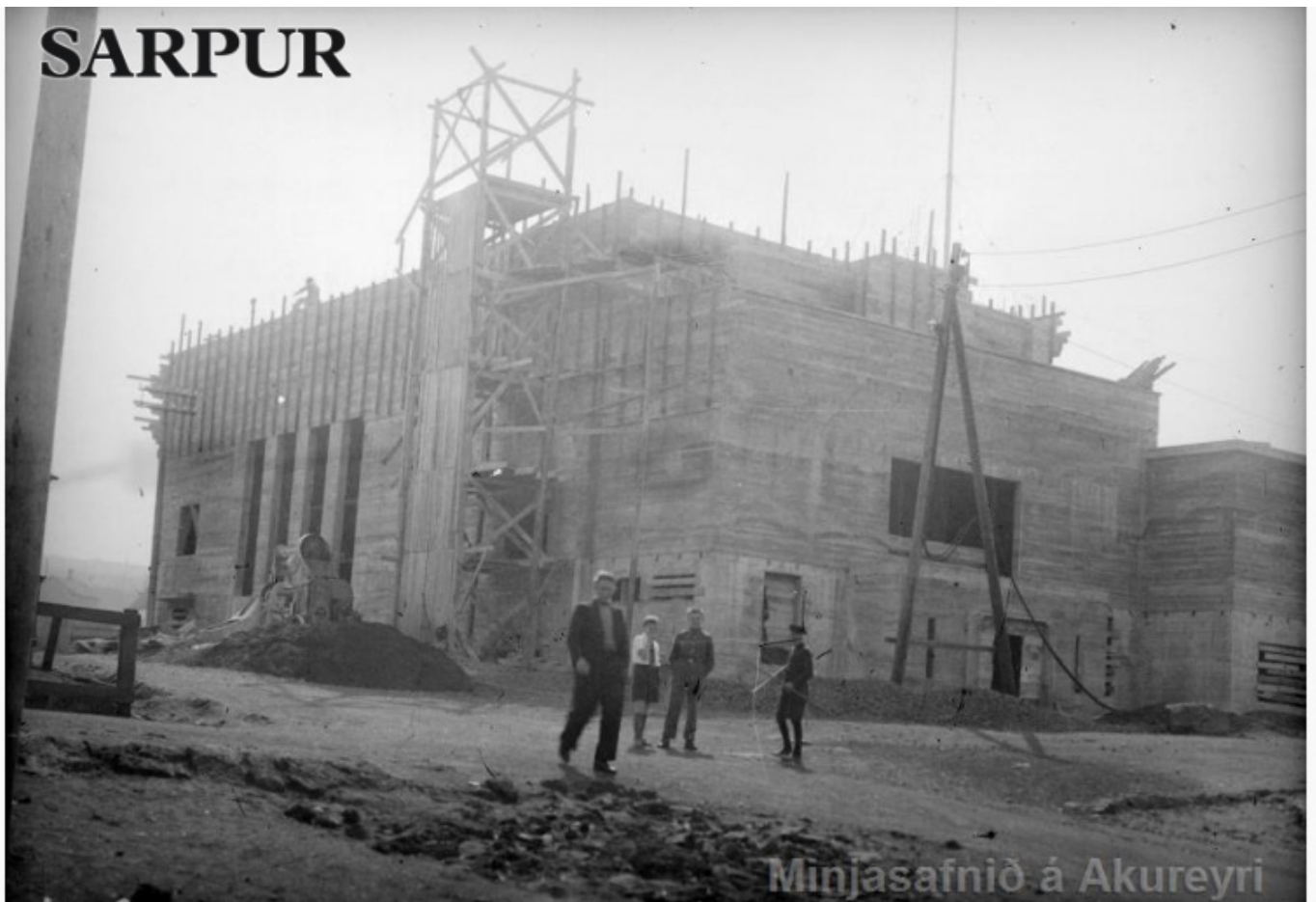
Fig. 33a–33b – The “formwork of Reykjavík” in use, ca. 1933–38. Borgarsveit (above) and the Westman Islands (below). Þjóðminjasafn Íslands/National Museum of Iceland.
