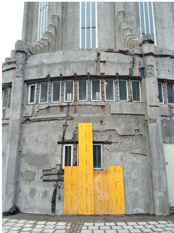
Fig. 13 – Renovation works on the church of Hallgrímur, Reykjavík. Photo by Sofia Nannini, 2018.
