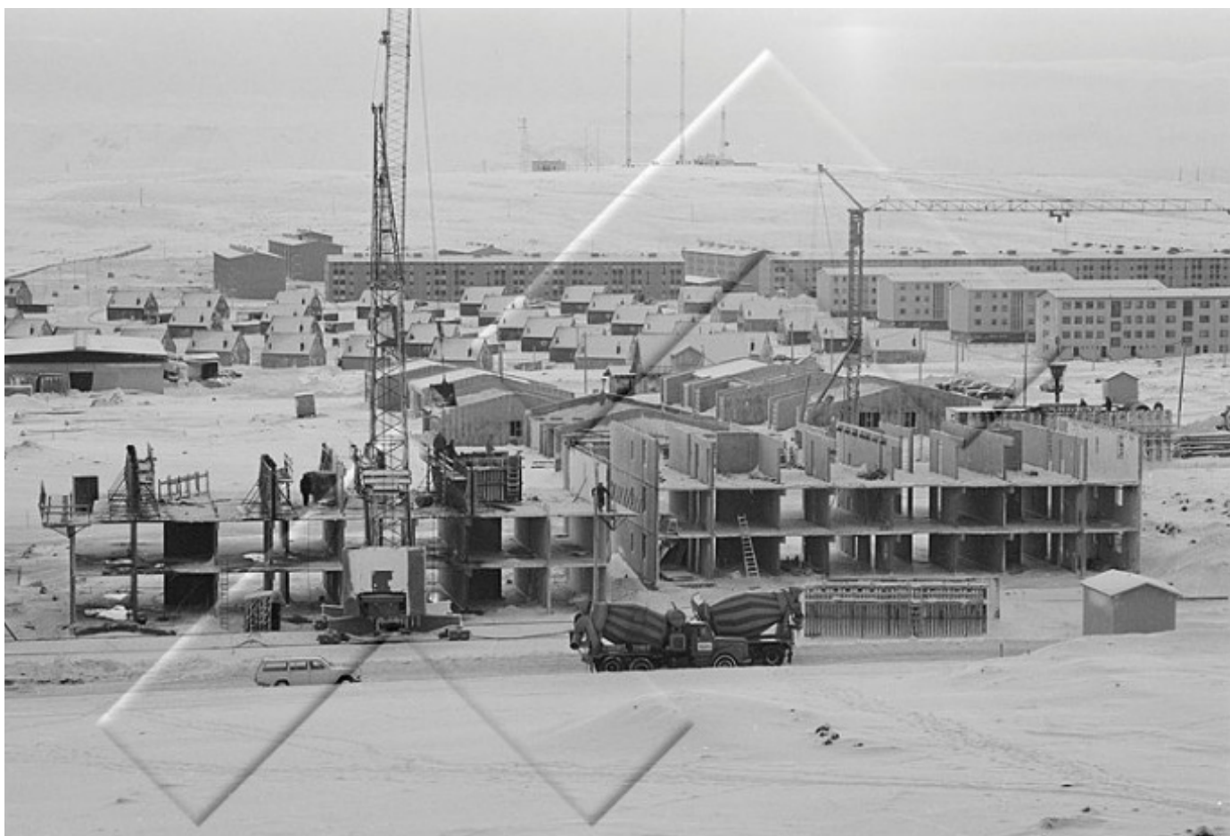
Fig. 3b – Residential units in construction, Breiðholt, Reykjavík, 1979. Ljósmyndasafn Reykjavíkur/Reykjavík Museum of Photography.
