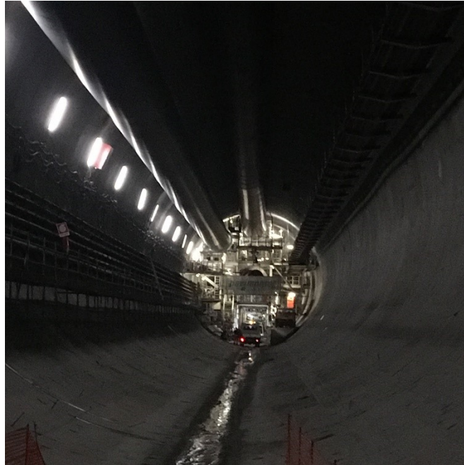
Figure 19 - Provision tubes are clearly visible on the left of the photo. The machine backup is depicted in the centre.
