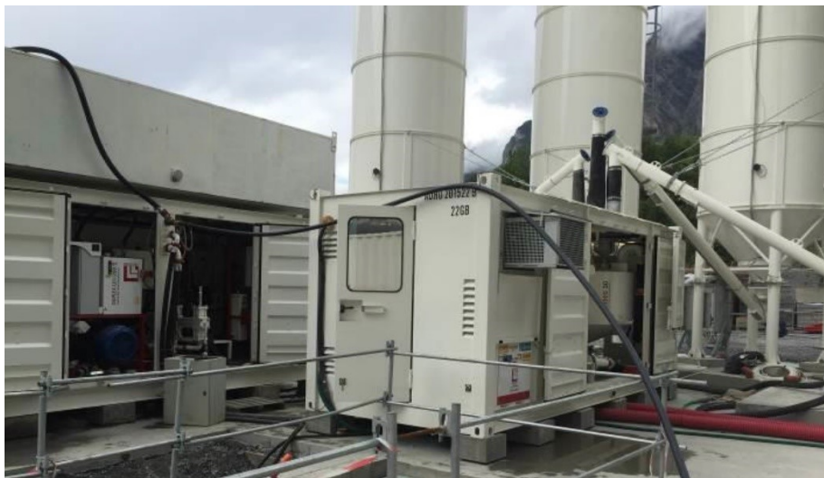
Figure 15 - Working site batching station. Mont Cenis base tunnel, France (Dal Negro et al., 2017).
