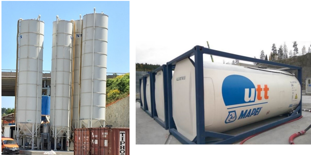
Figure 13 - Raw materials for the two-component grout production. On the left, the construction yard of the “Variante di Valico”, Barberino di Mugello (IT). On the right, tanks for the component B storage relating to the Follo Line project (NO) (Dal Negro et al., 2017).
