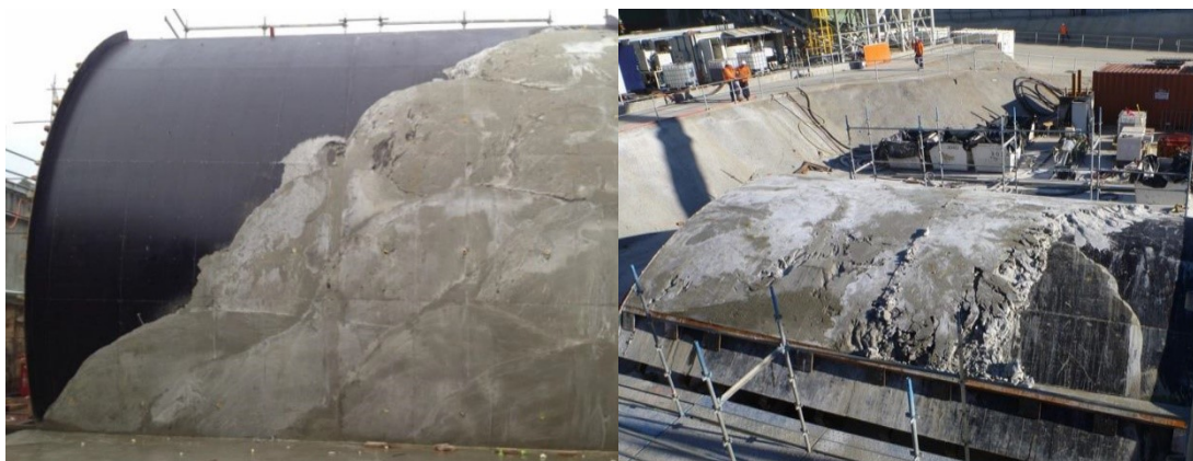
Figure 24 - Hardened two-component grout after the full-scale test. Injection at the inverter and on the lateral part (left) and crown injection (right) (Dal Negro et al., 2014b).
