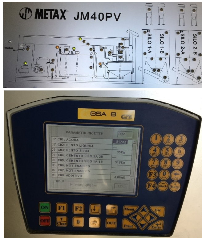
Figure 14 - Control panel of the batching plant and warning lights (top). Dosage setup display (bottom).
