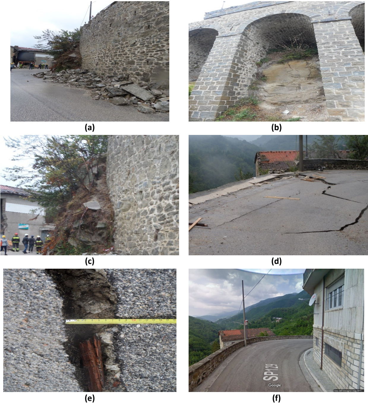
Figure 7.4. Masonry retaining wall in Arquata del Tronto (42.771898N, 13.296715E): (a) partial collapse of the wall parapet, (b) arch masonry structure, (c) marl blocks along the SP129 road, (d) road instability at the top of the wall, (e) opening of the cracks developing along the direction parallel to the road axis, (f) Google Earth view of the site (dated May 2011).
