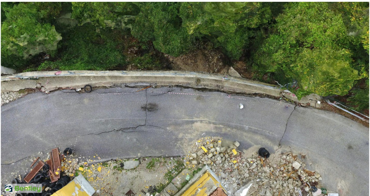
Figure 4.44. Rotated retaining wall below the road Frazione Fonte del Campo and subsequent cracks up to 25 cm in width (42.69438 N 13.24995 E).
