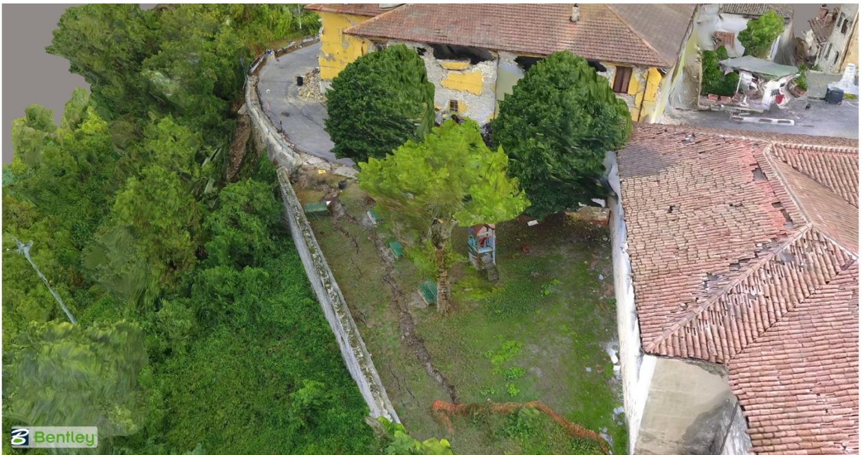
Figure 4.42. Model image of a rotated retaining wall (3.5-degrees) and the subsequent soil graben behind the wall (42.69446 N 13.24980 E).
