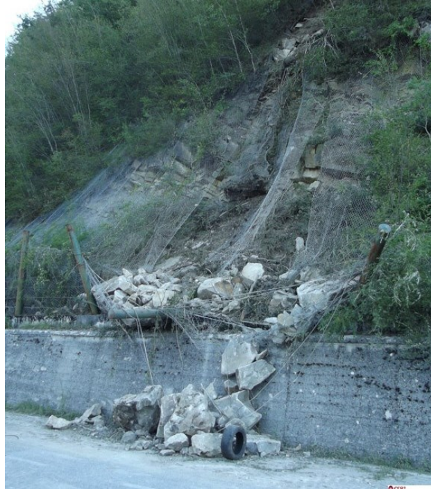
Figure 4.5. Rockfall involving sandstone slabs overlying marl layers (after CERI 2016).
