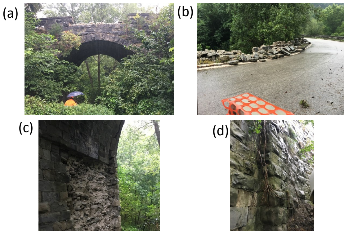
Figure 6.8. Central arch of the three arches masonry bridge along the Trisugo route (42.73538 deg, 13.253655 deg): partial collapse of the railing (a, b) spalling (c) and cracking (d) of some masonry elements.
