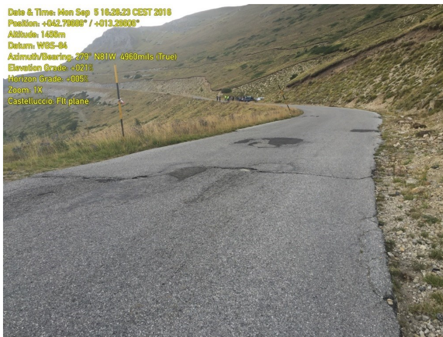
Figure 2.19b. Mt. Vettore fault: Damaged asphalt on SP477 at the fault crossing with less than 10cm of normal displacement down toward the west. Displacement are masked by bridging of the asphalt surface (Latitude and Longitude are annotated on the image).
