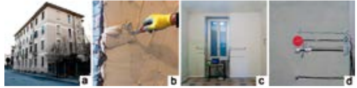
Figure 3 – a) The ATC building selected as pilot site; b) the plaster application; c) the walls selected for the monitoring; d) the sensors adopted for the monitoring
