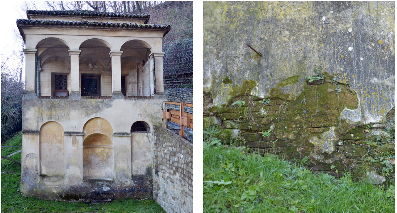
Fig. 2. Serralunga di Crea, Sacro Monte, Chapel 1. Main façade (right) and damage at the base of the northern façade (left).
