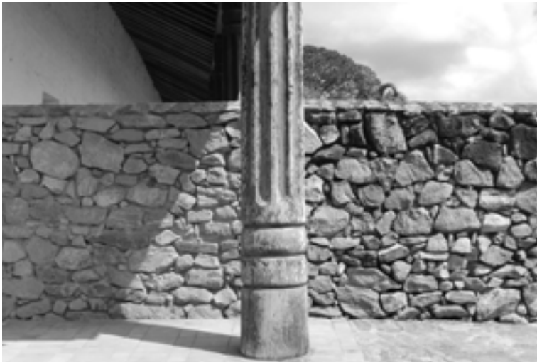
Buildings of the original complex of the Mission. Decay
