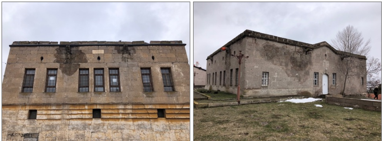
Figure 135: Lack of maintenance (author, 2019)
