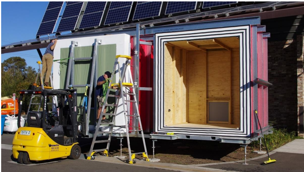
Figure 3.2. Assembly of the test cells. On the left, a test façade is being fixed to the test cell with the help of a forklift. On the right, the interior of the test cell.
