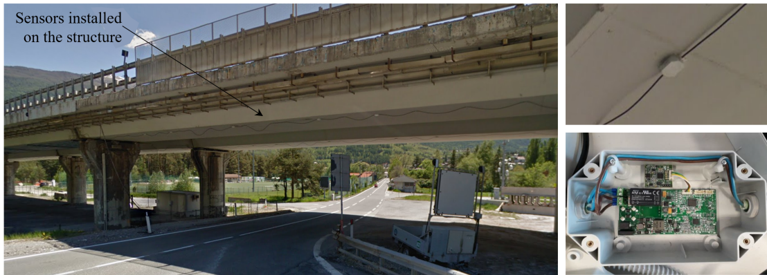
Figure 6.7: Sensors installed on the bridge
