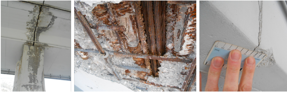
Figure 6.4: Damage evidences highlighted during visual inspections
