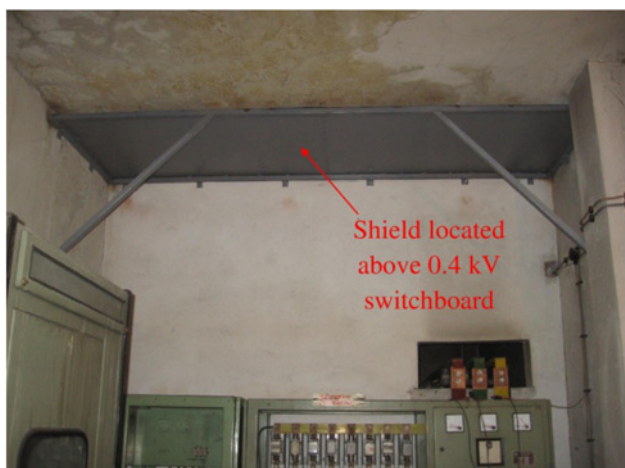
Fig. 6 Shield located above the 0.4 kV switchboard
