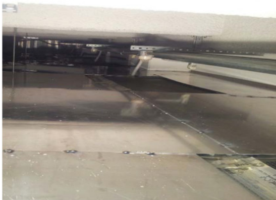
Fig. 14 Picture of the second shield: above the boxes of the power transformers
