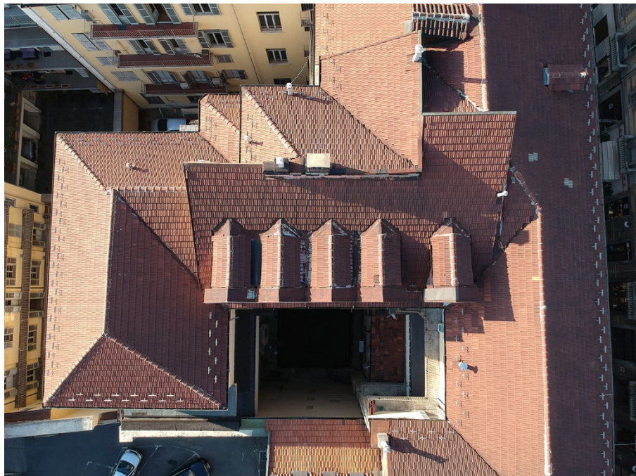
Figure 8. Picture that shows the roof system of the inspected building. The frame was taken with UAV's camera (source: real estate company archive).
