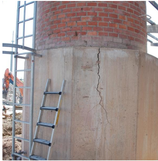
Fig. 3: Cracks in the chimney
