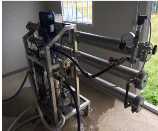
Figure 2.2: Picture of the nanofiltration pilot plant used to conduct the field experiments. The system was adapted to work with only one of the three pressure vessels available (stainless steel tubes), thus running each test with two 4040 membrane modules in series.
