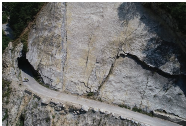
Figure 1. 2014 landslide's event which closed the SP 104.
