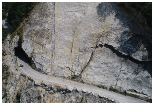
Figure 1. 2014 landslide's event which closed the SP 104.
