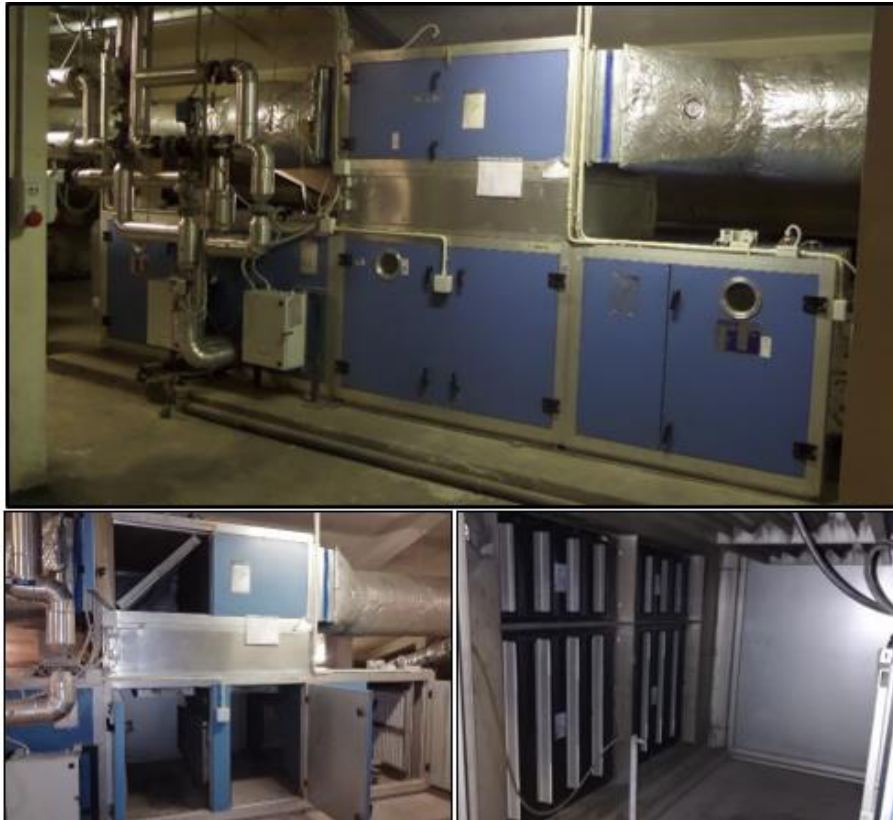
Figure 3 HVAC unit where monitoring the natural ageing of HVAC air filters.
