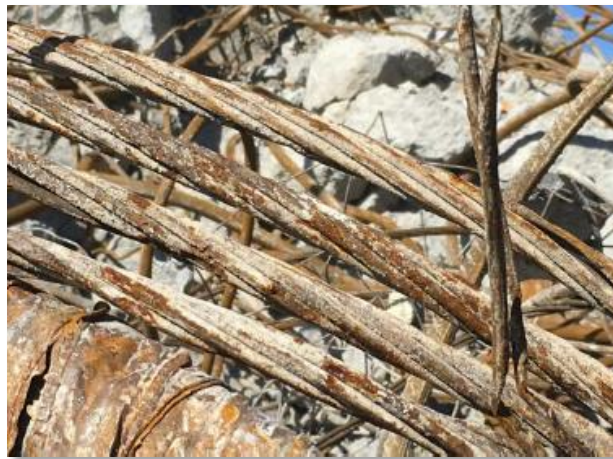
Figure 2. Pitting corrosion of prestressing tendons.
