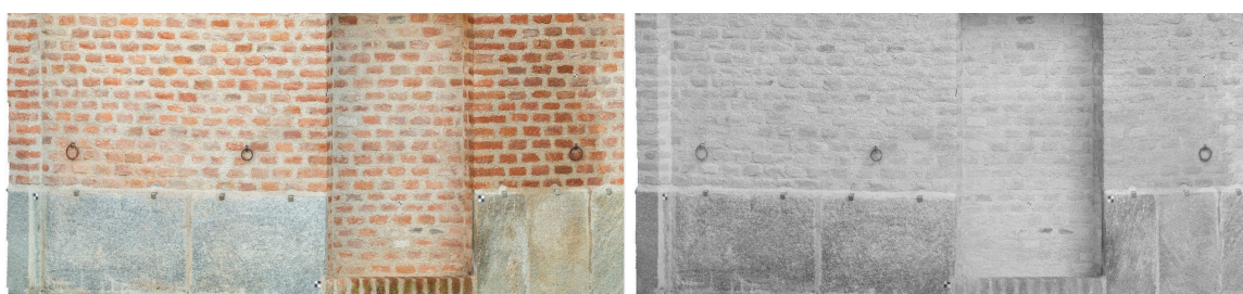
Figure 12. Comparison of details from the VIS (left) and NIR (right) dataset 2 textured models to evaluate identification of bio-deterioration on the façade's surface.
