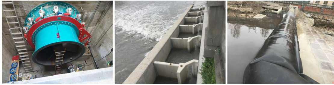
Fig. 10. The first picture show the positioning of Kaplan Turbine, the second one shows vertical slots of fish pass and the third one shows the inflatable check dam (Authors, 2017).
