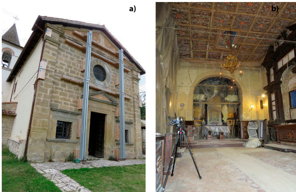
Figure 1. (a) Shoring works on the facade of the Sanctuary of Santa Maria delle Grazie at Varoni after 2016 Central Italy earthquake; (b) Interior of the single nave of the church.
