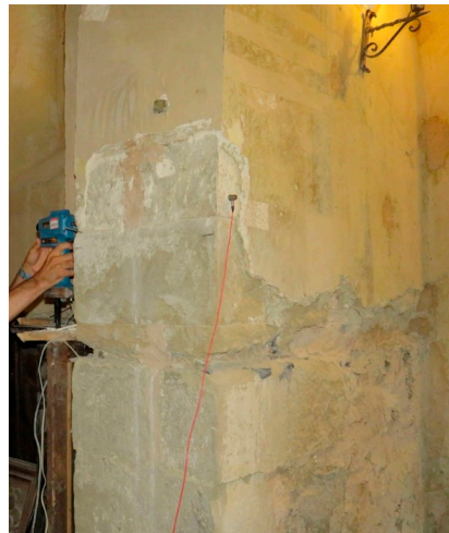
Figure 7. Impact test on single big sandstone constituting the masonry texture.
