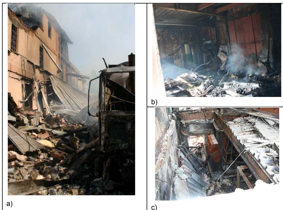
Figure 2. Damage of the main building from the exterior (a) and inside the A area (b,c).
