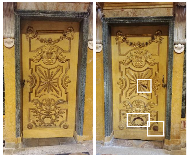
Figure 3a and b. The reference door used for the survey (left) and the ruined one (right) with the identification of the missing elements.
