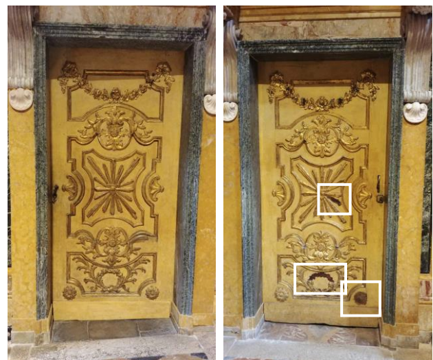
Figure 3a and b. The reference door used for the survey (left) and the ruined one (right) with the identification of the missing elements.
