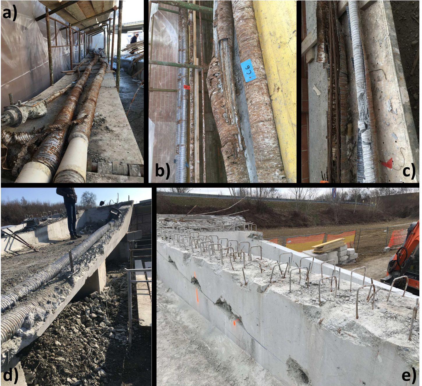
Figure 3: a,b) oxidated cables. c) in situ casted cable. d) dissection and extraction of one of the main cables. e) extracted stirrups
