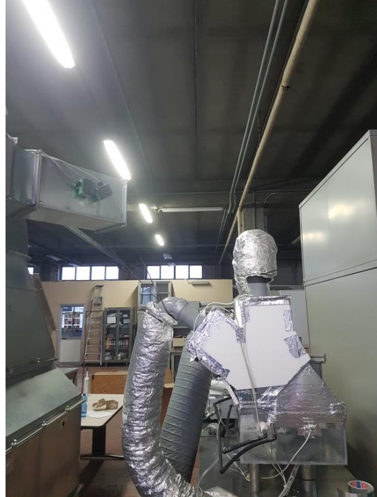
Figure 5. Condenser and heat recovery system
