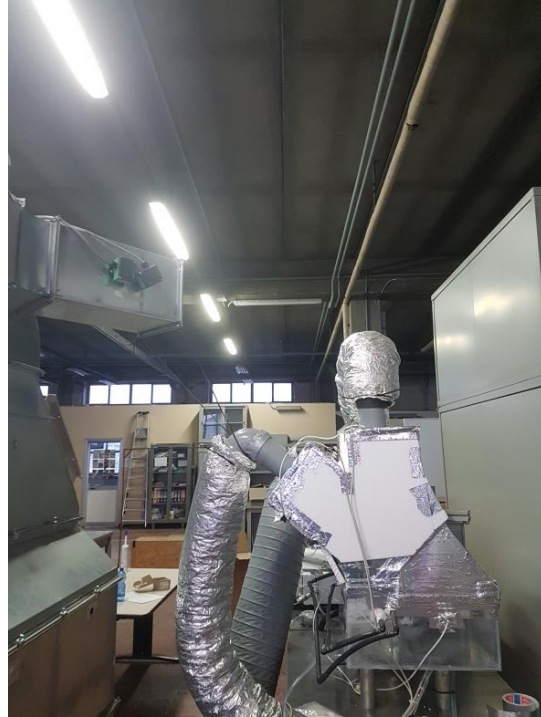
Figure 5. Condenser and heat recovery system
