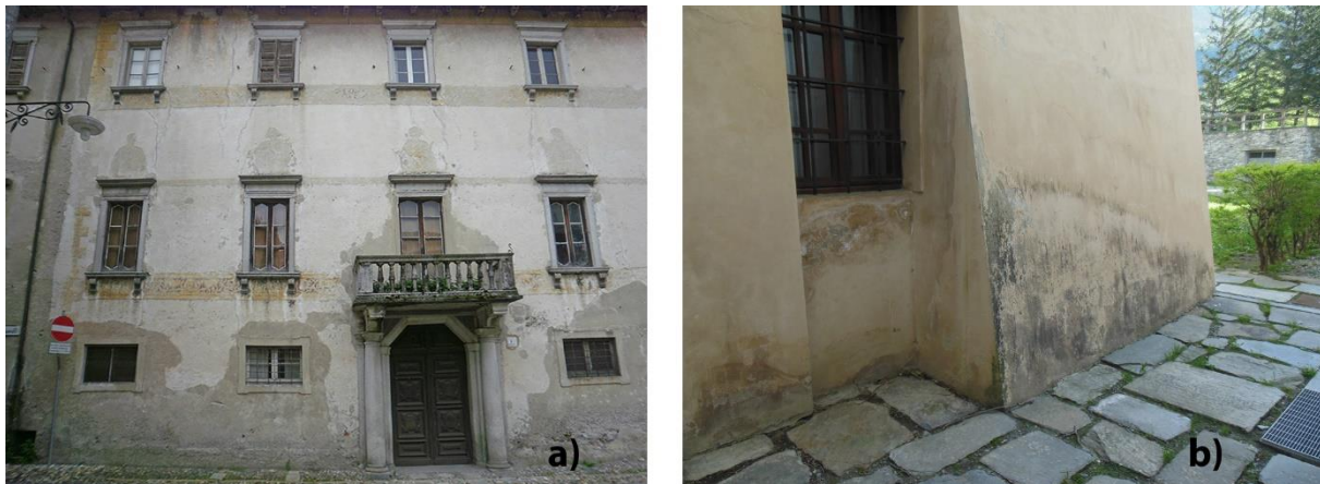
Figure 1. (a) Patches of cement/lime based plaster on historic façade; (b) deterioration (with detachment) of cement plaster applied for the restoration of a masonry subject to moisture.
