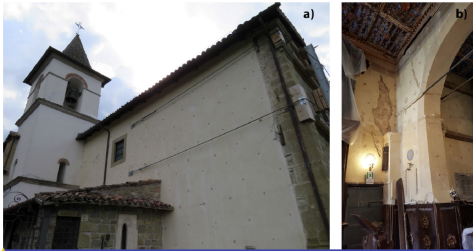
Figure 10: (a) Signs of the execution of reinforcement injections on the walls of the church; (b) second iron tie carried out in pairs with the one existing at the triumphal arch.
