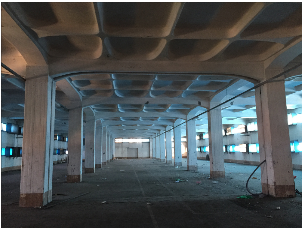
Figure 6: Concrete slabs of the 'Ballette' Building, Manifattura Tabacchi, Bologna. Photo by Micaela Antonucci, 2017.
