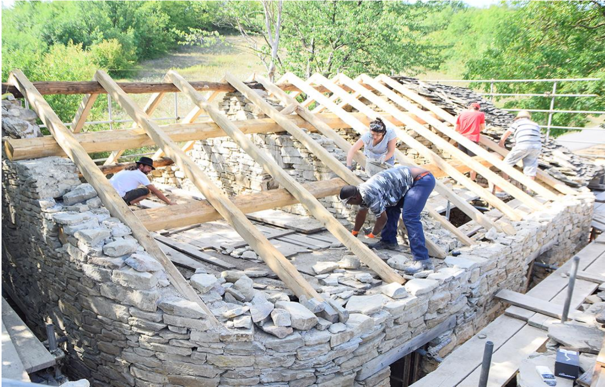
Figure 1. Banca del Fare summer workshop. Students and experts are working side by side in restoring a vernacular stone building. ©Banca del Fare
