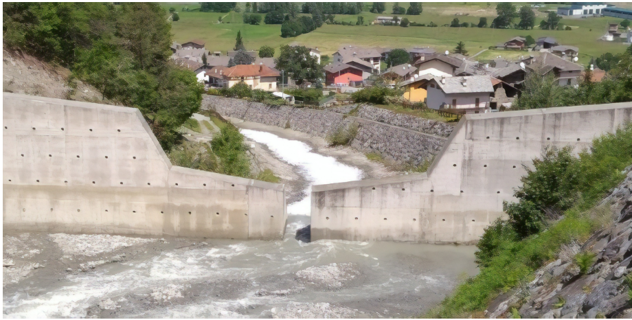
Fig. 1. A debris-flow retention structure located in Pollein, Aosta Valley autonomous region, Italy.
