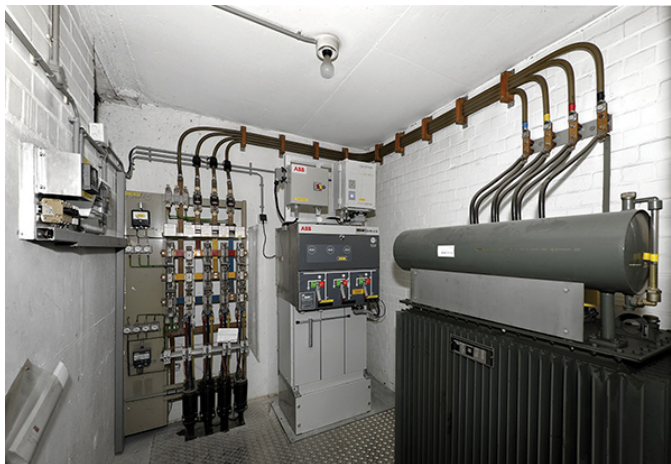
Figure 3. Typical indoor MV substation. Image taken from http://electrical-engineering-portal.com/
