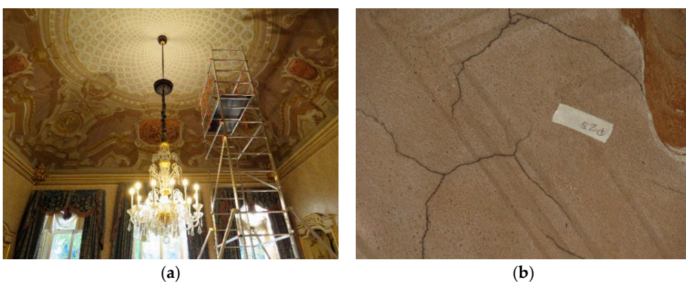
Figure 3. (a) Giunta room at Birago Palace; (b) cracks branched in the decorated plaster of the masonry vault in the Giunta room.
