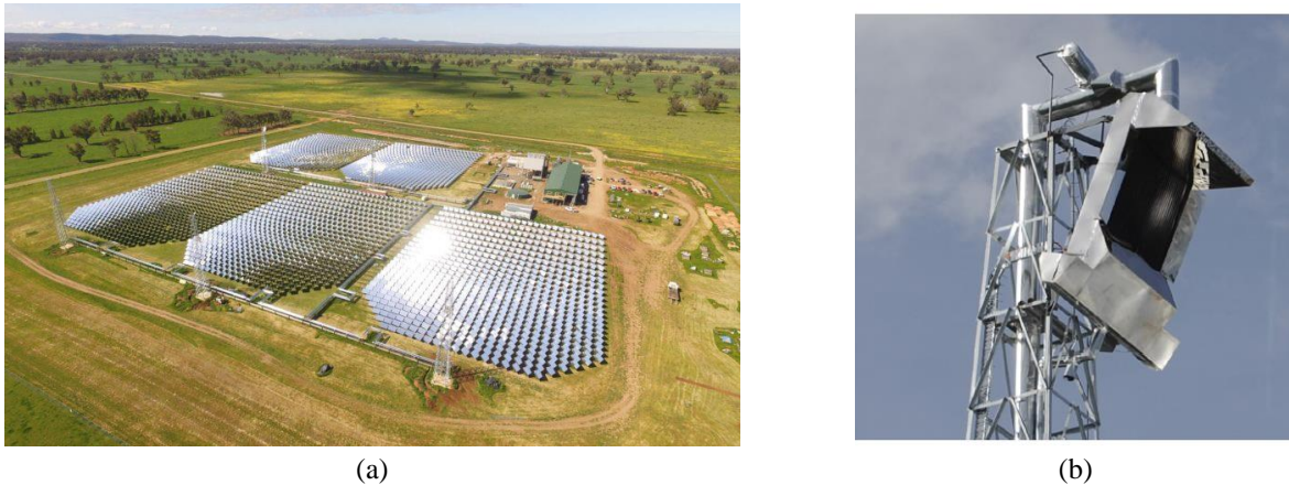
Figure 1 – Jemalong Solar Thermal Station, (a) aerial view of the whole plant and (b) solar receiver
