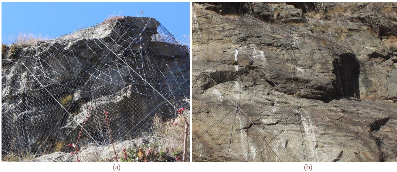
Figure 6: In (a) two mesh types are adopted; in (b) the simple and the reinforced drapery systems are adjacent in the same site.
