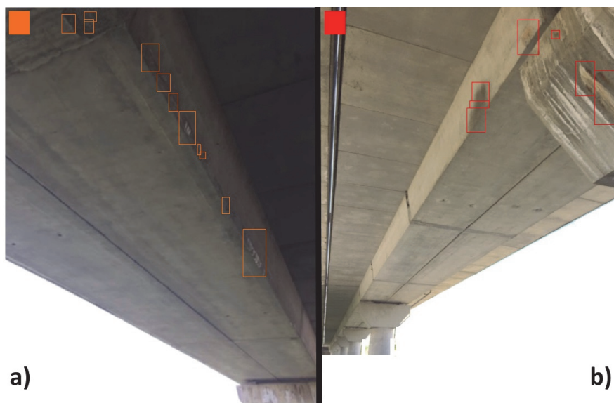
Figure 24: Detection of a Lv.3 damage (a); detection of a Lv.4 damage (b).
