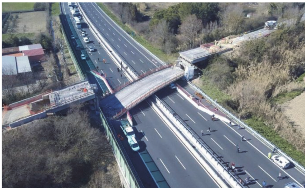
Figure 6: Ancona overpass after the collapse (from web site www.cronacheancona.it ).
