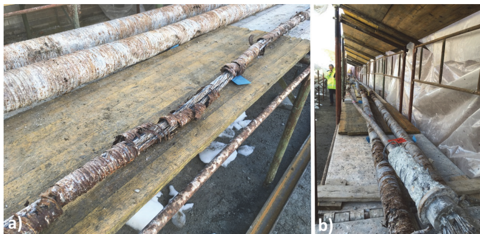
Figure 10: prestressing cables, extracted and analyzed. It is possible to note the direct correlation between grout content and oxidation rate of both sheathing and strands.
